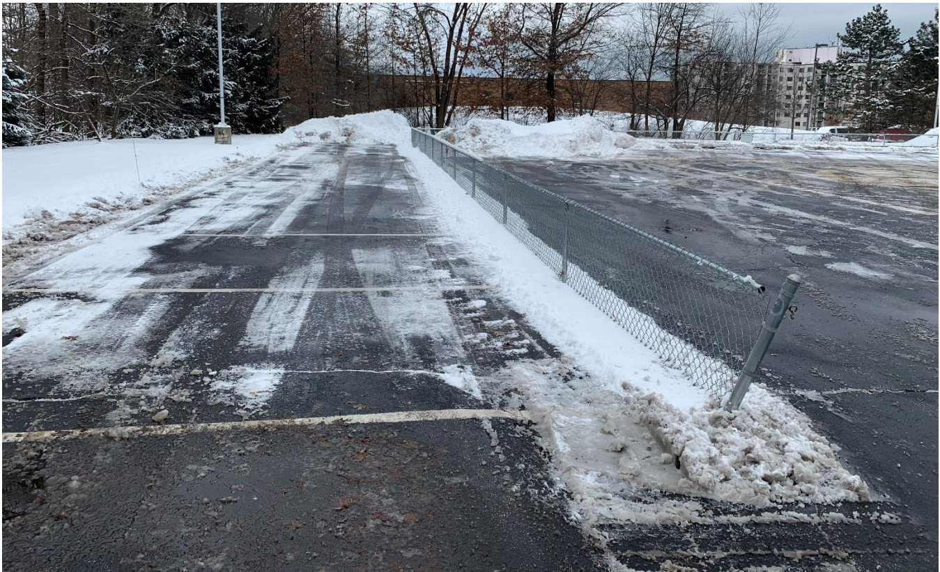
Figure 2: Helipad Placement Inefficiencies
